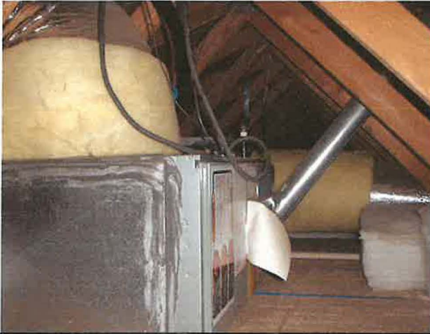
The Habitat replacement furnace
