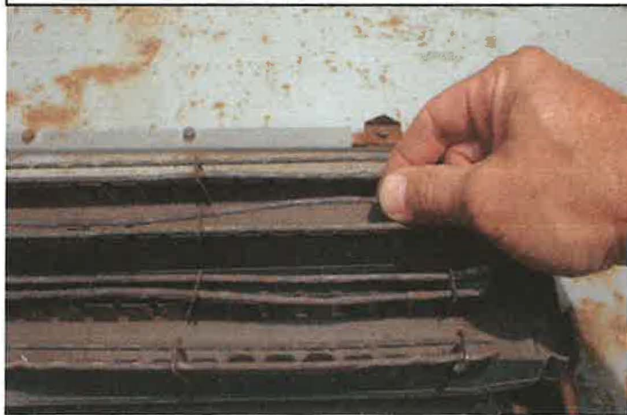
NOx rods on the Habitat furnace were clearly fatigued
