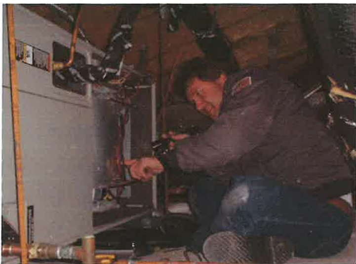
Service Manager Ralf Kies prepares to measure wet and dry bulb temperatures across the air handler.
