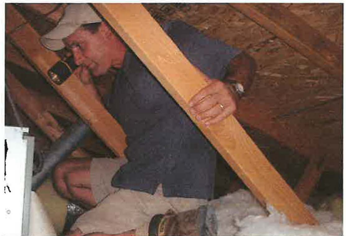
Checking flame conditions for ruptured heat exchanger
