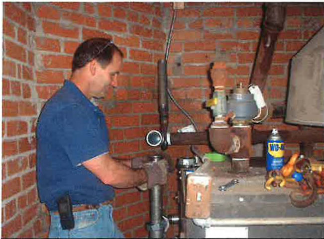
Preparing to replace a check valve and install a condensate pump and receiver
