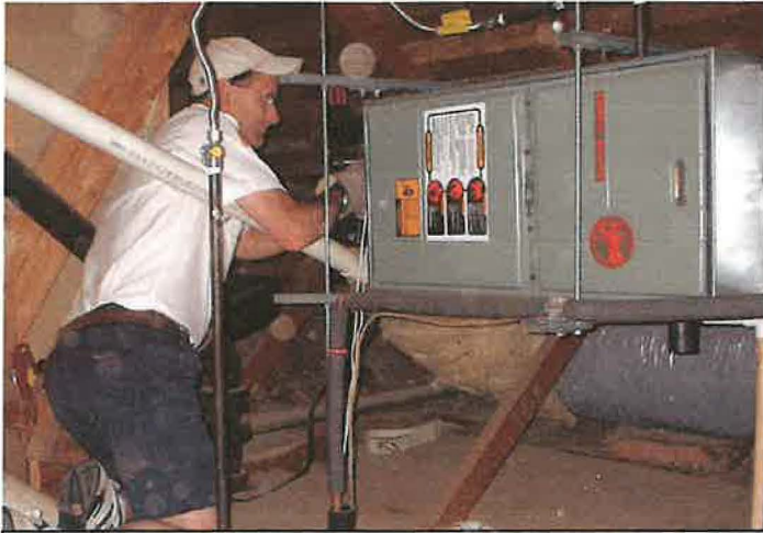
The Bender replacement furnace was hung away from combustible material
