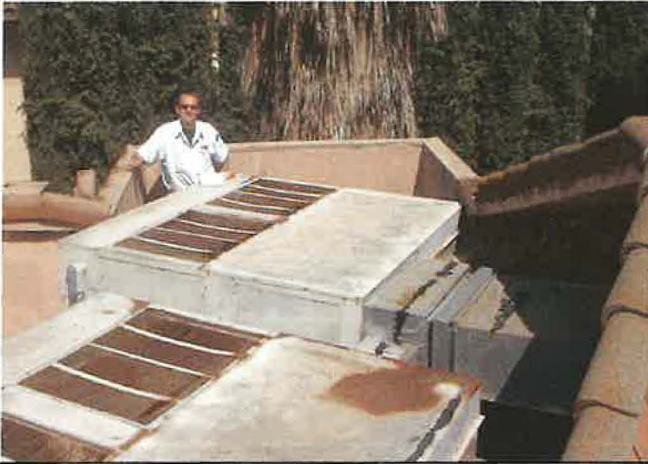
Two ten ton package units served the sanctuary at the First Methodist Church in Walnut, CA.
