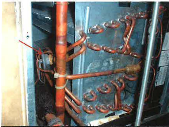
The metering device is often deep in the equipment and difficult to repair.
