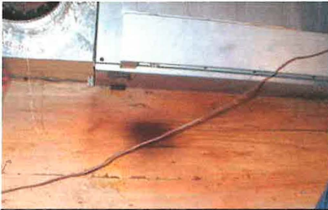
The Bender furnace showed signs of flame roll-out caused by a cracked heat exchanger
