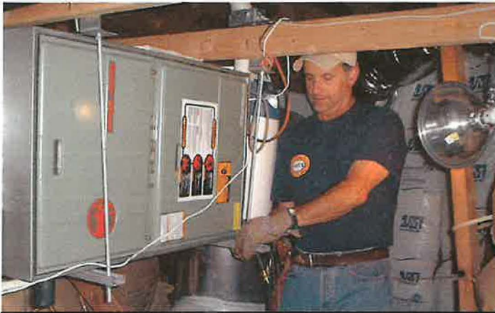
The Corydon furnace was hung from rafters and hard duct attached to the existing air distribution system
