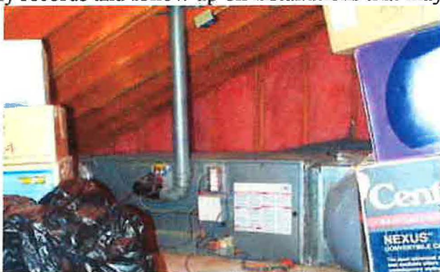
The Bender furnace was located dangerously close to combustible material
