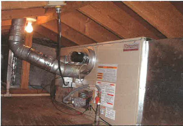
The Gant attic space was too confined to hang the replacement furnace
