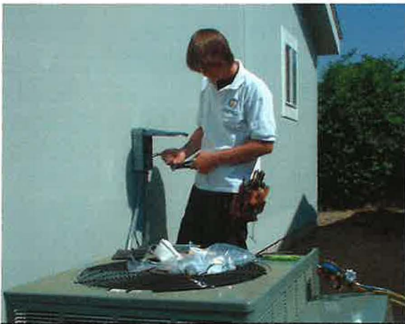
The electrical disconnect is installed
