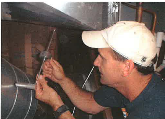
The counter weight is set on the bypass damper
