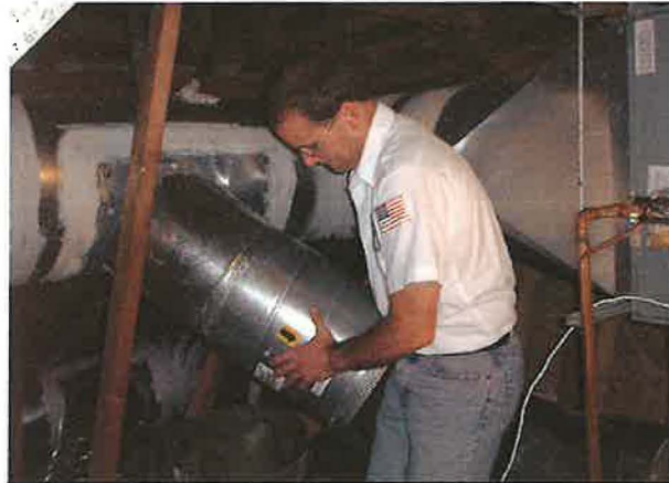
The bypass damper is installed in the supply duct to relieve duct pressure during low loads
