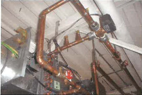
Reconfigured fan coils
