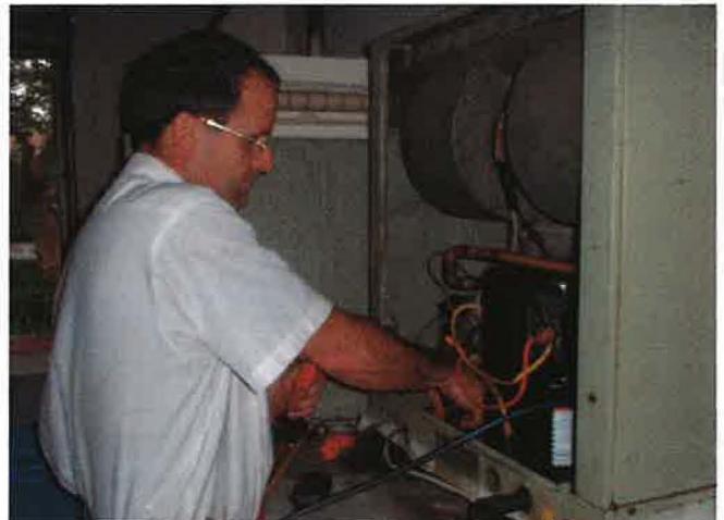
Checking the electrical windings of a hermetic compressor
