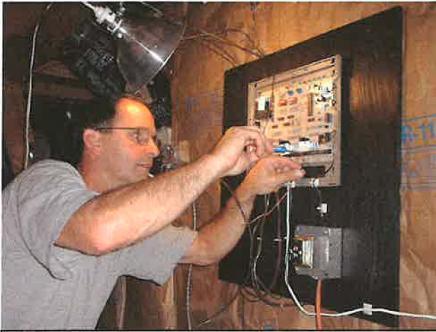
Zone thermostats are connected to the TZ-4 control panel
