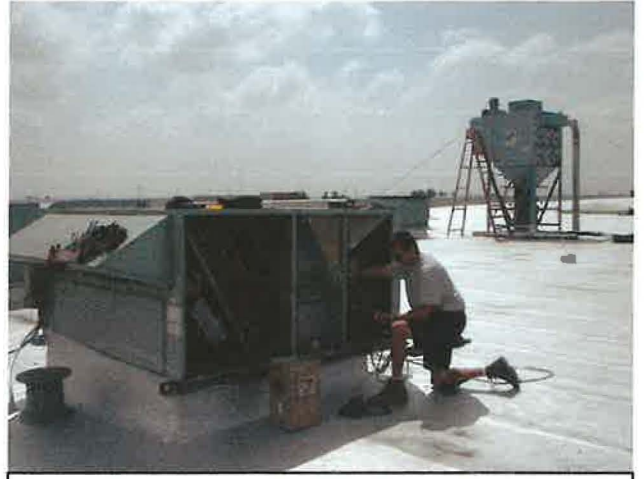
Checking the operation of package air conditioner
