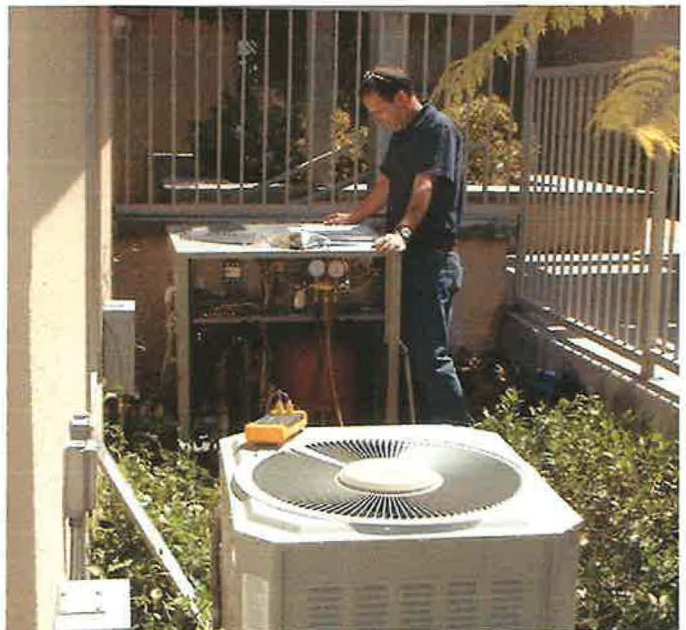
Two 3 ton air conditioners are checked for saturation temperatures, superheat and subcooling.
