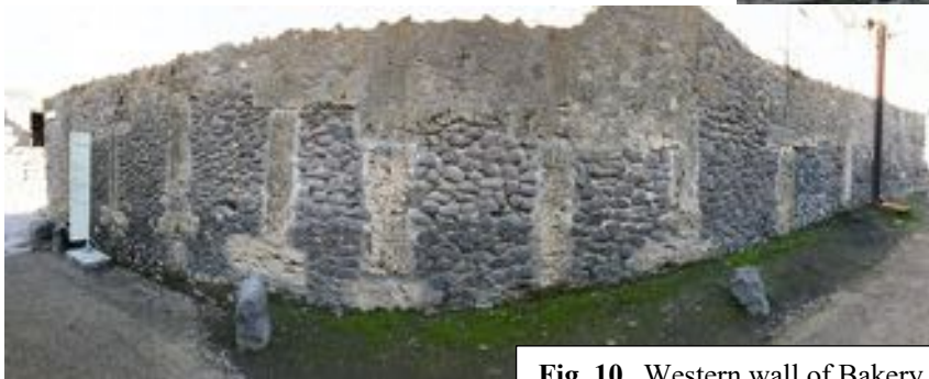
Fig. 10 Western wall of Bakery I.12.1. Travertine and lavastone opus africanum , on the Vicolo del Nave Europa, Pompeii. (The curvature in the wall is an optical distortion resulting from the panoramic photograph.)
